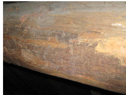
Purlin in roof space with worm.
